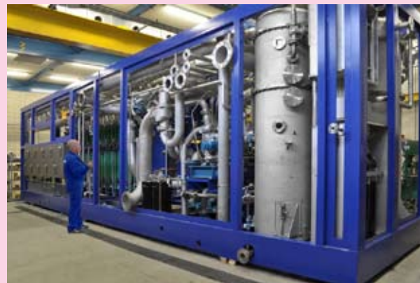
Figure 14 1 MWe – PEM Power Plant at Solvay, Antwerp
