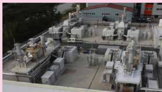
Figure 8: Daegu, 11.2MW MCFC installation in Korea
