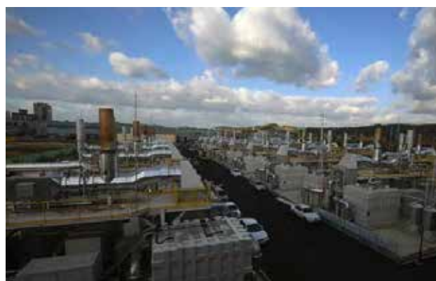
Figure 7.2: The world's largest MCFC power plant located in Hwaseong City (Source: POSCO Energy)
